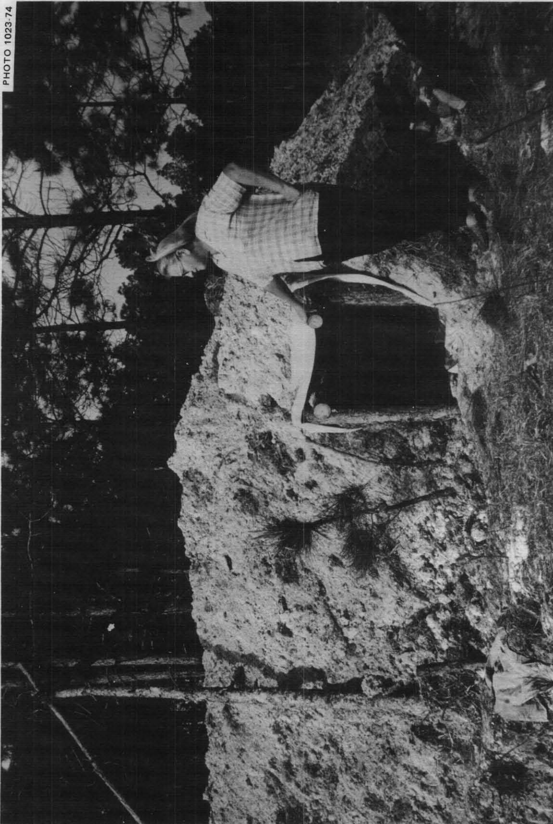
Fig. 5.52. The properly completed entryway of the A-Frame Pole Shelter, pictured on the day following its completion. These hard-working rural families built this 21-person shelter in 12 hours 14 minutes, from the time they received the instructions on a farm about 2 miles from the shelter-building site.
